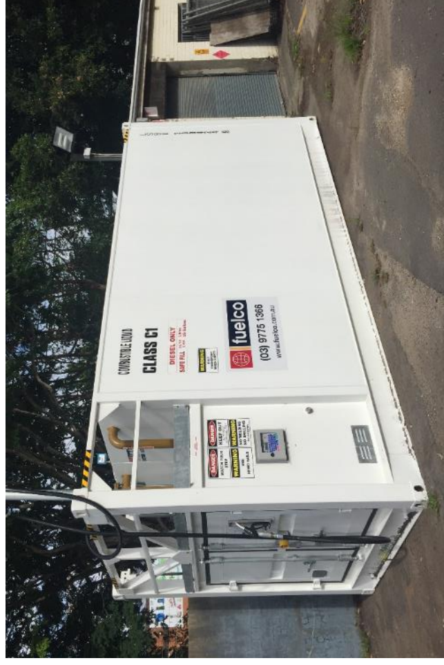
Image: New installation of bulk fuel tank at Parks Nursery St. Peters
