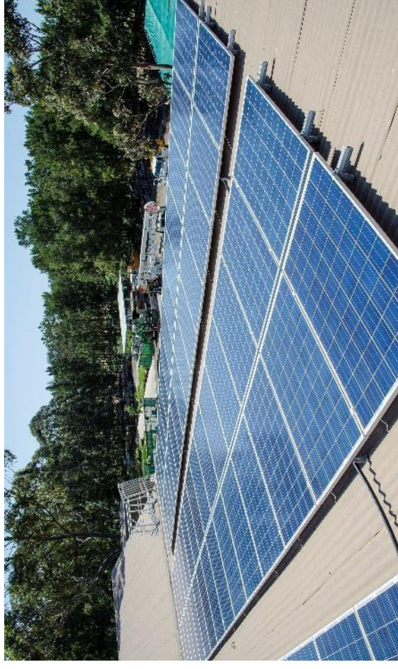
Image: Solar PV panels at Sydney Park Nursery
